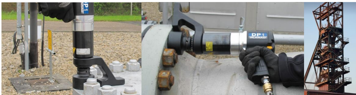
Fastening of blanking caps and pipe flanges on a gas compressor station with the pneumatic torque wrench DP
